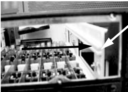
Example of an empty bay. Note guide rails along the inside edge
